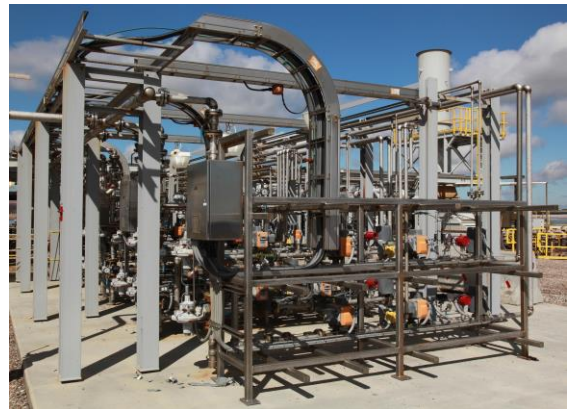
Fuel Safety and Control Trains
